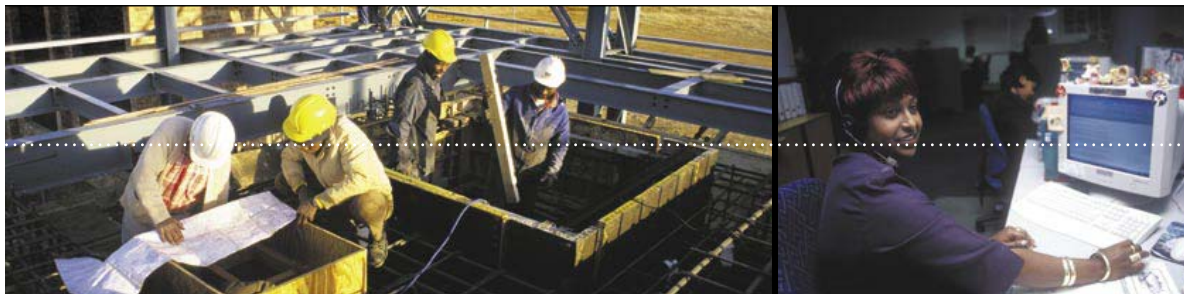
A construction site at a mine in the Free State. The development of artisan and technical skills for infrastructure development is a medium to longer-term objective of JIPSA. Photo: Graeme Williams/South Photos/The Big Picture.
