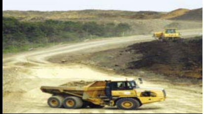
A road building project in the Eastern Cape. The development of artisan and technical skills for infrastructure development is a medium to longer-term objective of JIPSA. Photo: Peter Iturza/Alamy/The Big Picture
